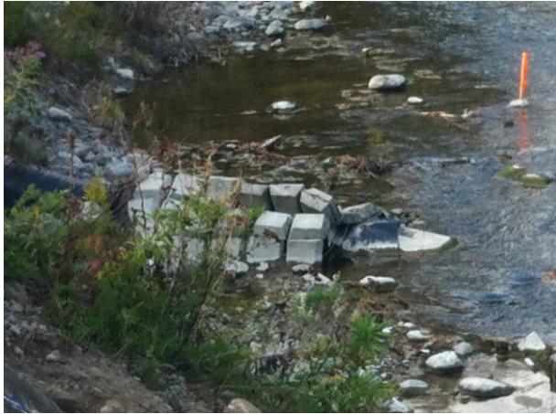
A dangerously exposed part of Line 9 in the Rouge River near Steeles & Morningside, Toronto, 2011.
